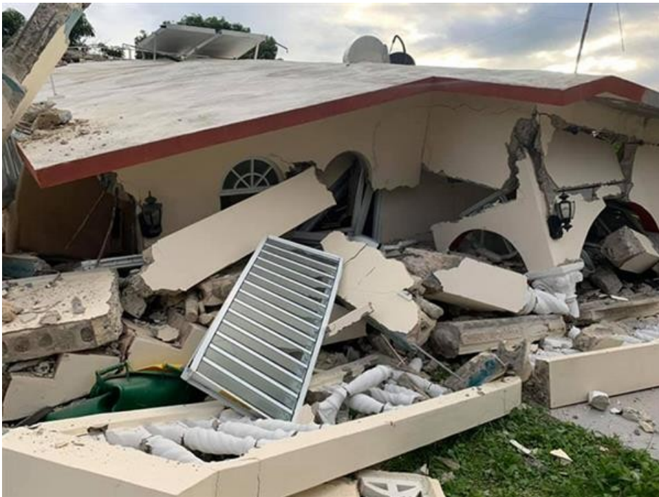
A home in Guayanilla, Puerto Rico, lies in ruins following a series of earthquakes. Hundreds of homes along the island's southern coast were destroyed or severely damaged, leaving many people afraid to sleep indoors. Photo courtesy of the Methodist Church of Puerto Rico.
